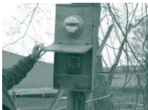
This is a fuse block device where you pull the handle which removes the block where you may need to replace the cartridge type fuses.
