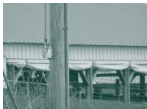
Remote switch for a pole top disconnect device. To reset, pull the lever down to the off position and push back up to the on position.
