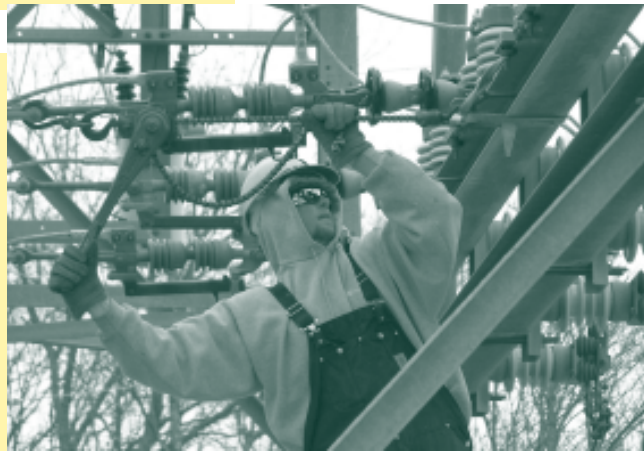
Hawkeye REC lineman Zach Steinmetz working at the Saratoga substation.
