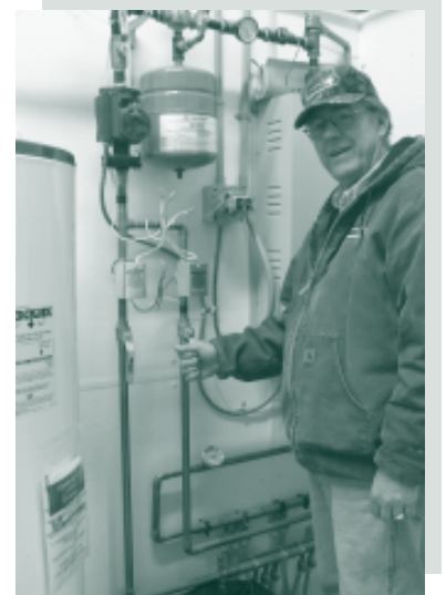
Hawkeye employee Wayne Kirkeby checks on the 9kW mini-boiler.
