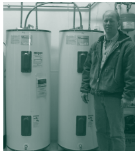
Hawkeye employee Marc Mikkelson with the water heaters installed at M & C Dairy in Lime Springs.
