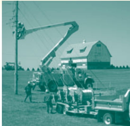
Crews continue to work on rebuilding 3½ miles of distribution line west of Cresco on Highway 9. This new line will tie four substations together, enabling Hawkeye to have greater reliability.
