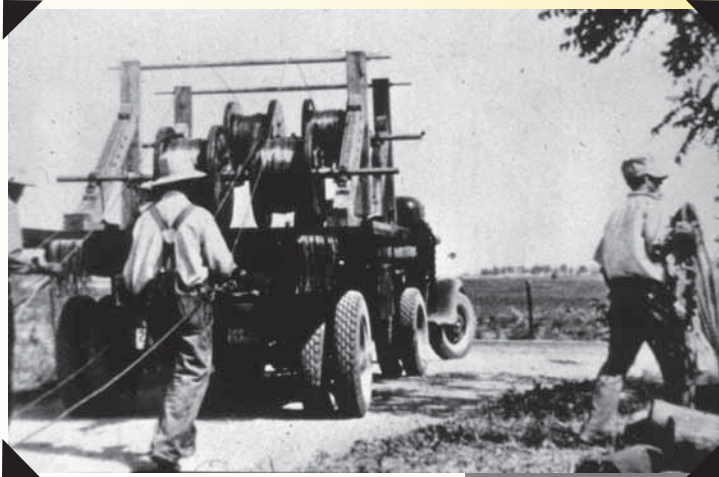
REA crews would have to string wires connecting the poles to provide electricity to the rural farmsteads.
