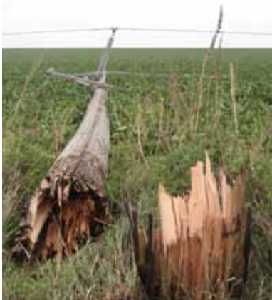
Over 67 structures on Dairyland Power's 3-phase transmission lines were knocked down.
