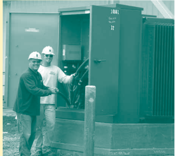
Hawkeye Linemen Wayne Hageman and Zach Steinmetz work on the large transformers equipped specifically for the Homeland Energy Ethanol Plant. Hageman was responsible for organizing the equipment and making sure everything was in place to ensure smooth operation at the ethanol plant.
